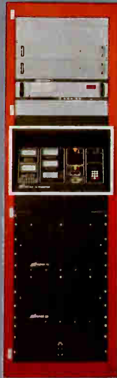
Front View with Doors Removed
