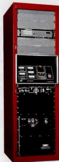
Driver Cabinet — Front, Door Removed
