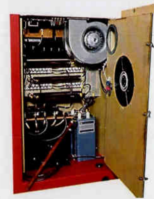
Driver Cabinet — Rear View, Door Open
