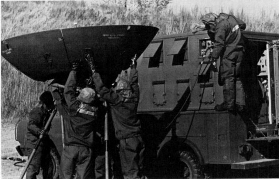
Members of the 5th Combat Communications Group complete installation of an eight-foot parabolic dish antenna at Eielson Air Force Base, Alaska during Exercise JACK FROST 79. The antenna is part of a wide-band radio system that provides communications services for other Air Force units in the exercise. (U.S. Air Force Photo by Major Carl F. Freeman)
