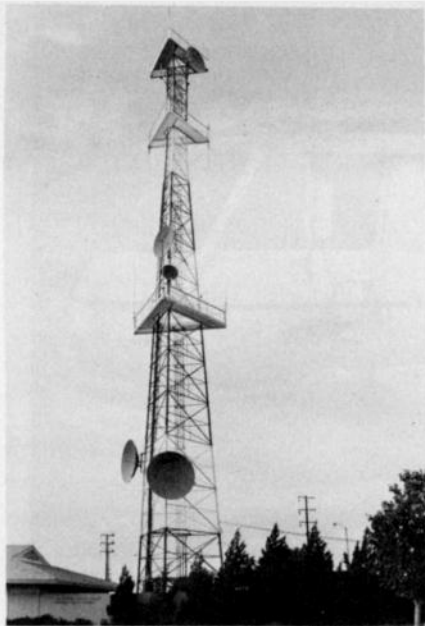
One single tower at a federal installation can be the location of many antennas generating signals on a large number of frequencies in all scanner bands, plus microwave!
