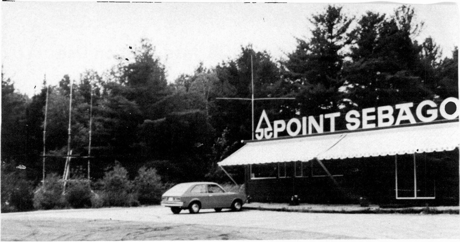
Photo 2—Installation of the Array at the Point Sebago Base Station. Antenna elements at the left of the picture form the new phased array. The single antenna formerly used is shown in center photo.
