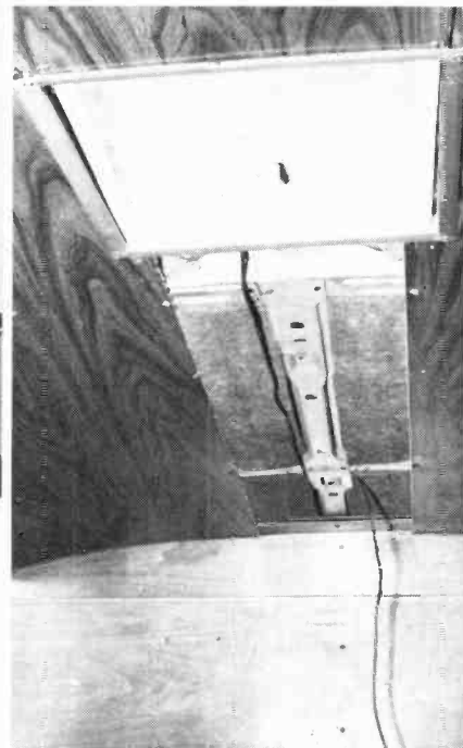
Connect the coax to the antenna mount and run it along the open area where the paneling has been removed.
