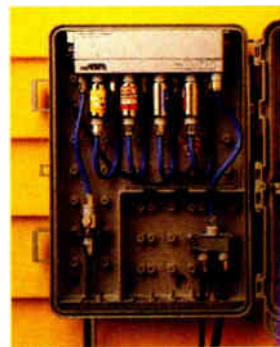
Fully-configured STARPORT unit within an on-premises enclosure.
