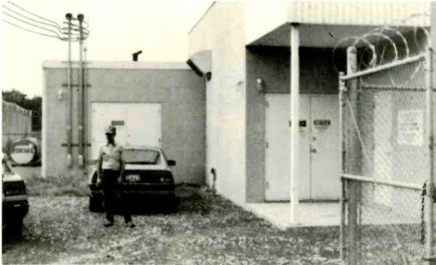
Building exterior showing security fencing, diesel generator area, and the transmitter exhaust duct.
