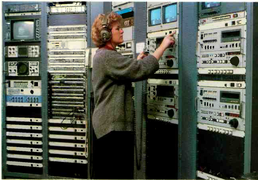
Machine control interfaces may be grouped together, or located at the individual machines.
