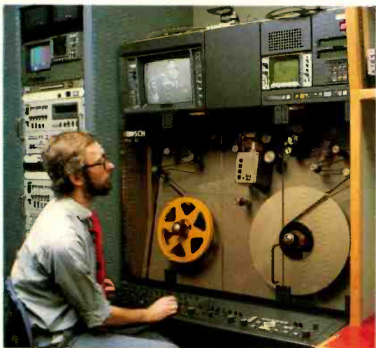
Projectors and telecine transports can be remotely controlled.
