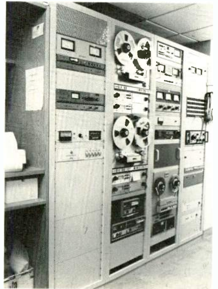
Common equipment racks in the hall outside of Studio A and Studio B.
