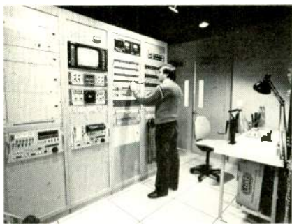
Machine room has film editing equipment in addition to Betacam recorders, Ultimatte, and test equipment.
