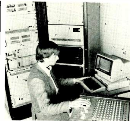
Gotham Audio's Systex audio storage system, showing HP host computer and audio console, in use at a broadcast production studio.
