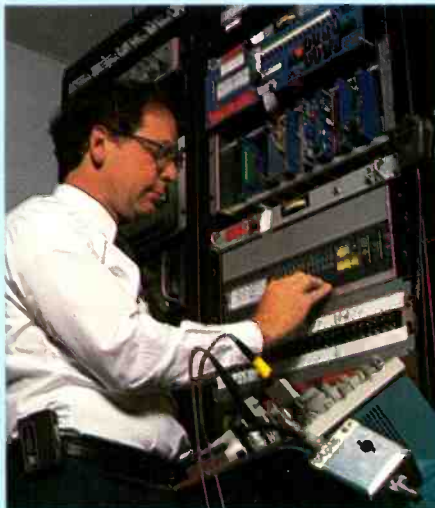
On October 15, 1984 at KTLA’s Mt. Wilson transmitter site, Ira Goldstone performed the final acceptance checks on the Modulation Sciences TV. Stereo Generator.
