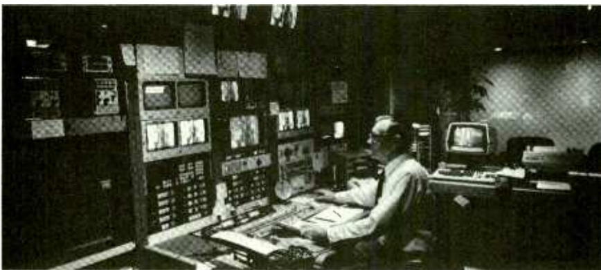
Master control contains a Vital VIX-115-4B switcher and remote controls for the RCA TTG-30/30L transmitter and Harris earth station.
