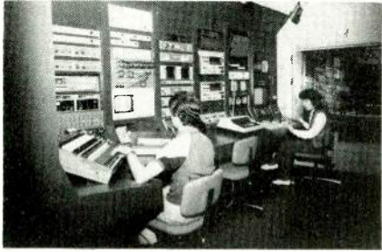
Control room at Continental Cablevision. Studio, seen through window at right, is often used for local shows.
