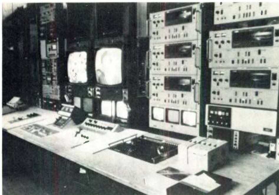
In master control, six U-Matics under microprocessor control provide majority of on-air signal.
