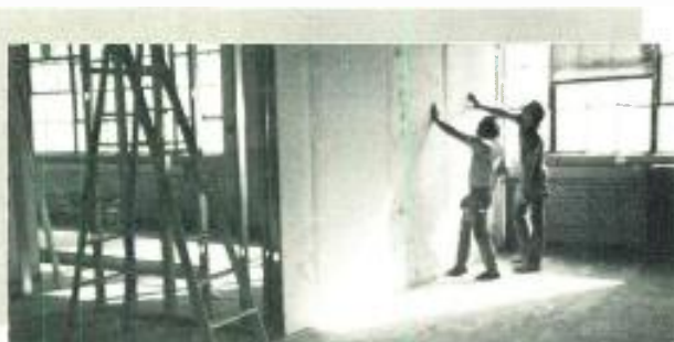
Workers install wallboard in offices that surround central working areas and studios.
