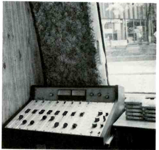
View showing the UFEI board at the engineer's operating position
