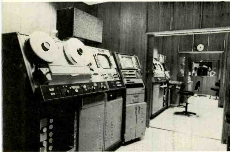
Videotape room at Sydney studios of Australian Broadcasting Commission, government's TV net, has Ampex VTRs installed in the changeover to color.
