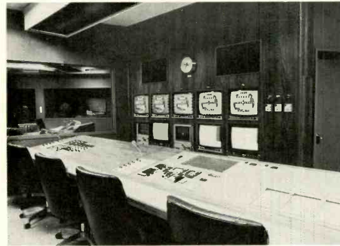
"Vision control" for large studio shows new cold switching equipment.
