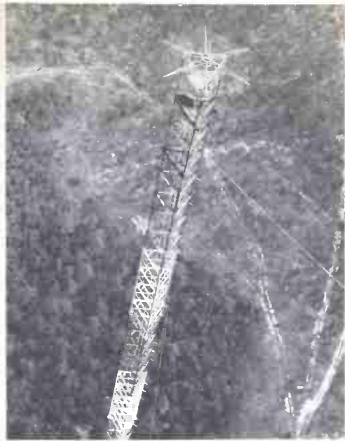
At Eglin Air Force Base in Florida, the 1200-foot communications tower has dissipation array at top. Rising out of flat land, tower used to be hit by lightning 100 times a year.
