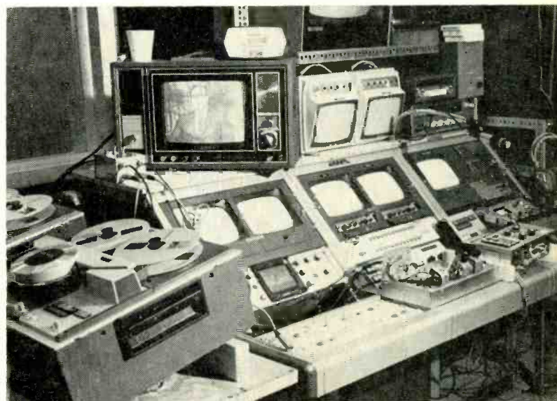
Twin County's control room. Uncased chassis is new synchronized switcher being built by staff.
