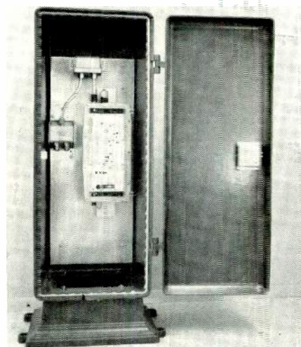
Entron uses Crouse Hinds Traffic Controller pedestal in their underground system in the Bronx. ●
