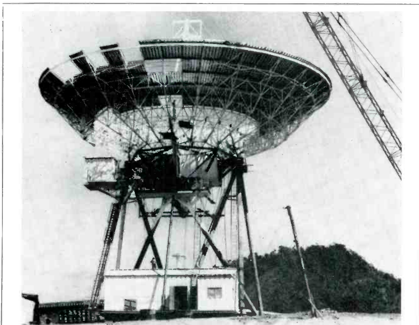
Construction of a multimillion-dollar satellite communications earth station is nearing completion in the Phillipines, it was announced by General Telephone & Electronics Corporation. Shown (above) is the station's dish-shaped antenna, measuring 97 feet in diameter. The station will serve as a ground terminal for voice, television and data communications to and from an Intelsat II satellite in synchronous orbit 22,300 miles over the Pacific Ocean. The station is located at Pinugay, about 25 miles east of Manila.
