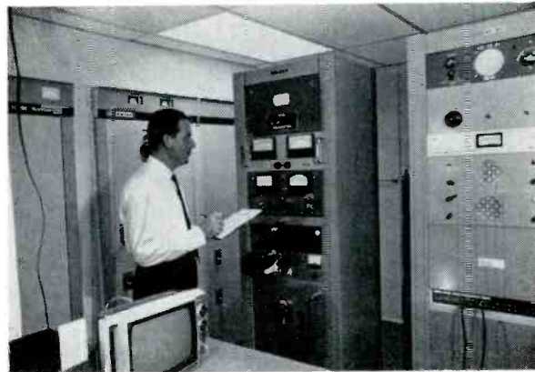
Main transmitter room contains microwave gear and 10-kW solid-state Gates BC 10H.
