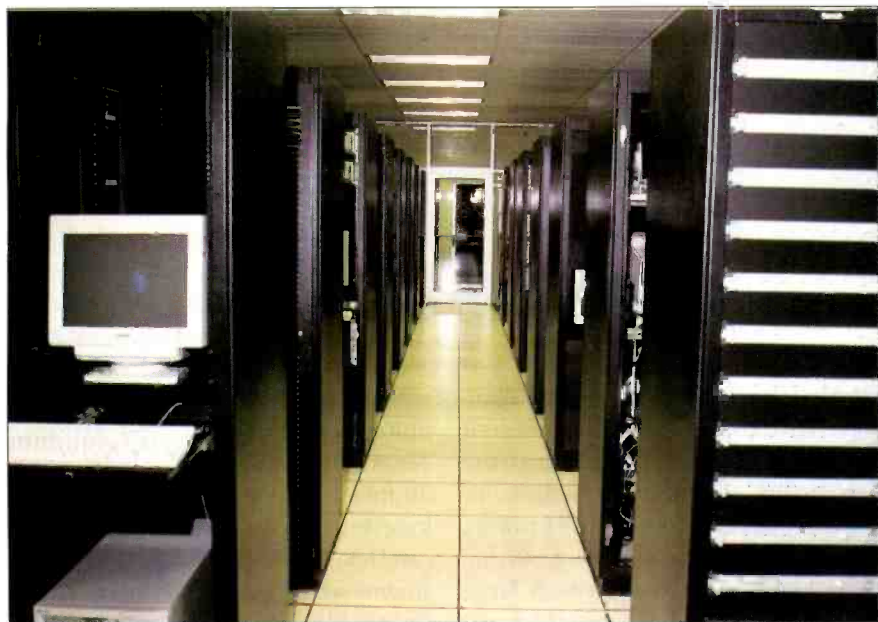
Main corridor through WSB's technical center, which houses 100 racks of support equipment.
