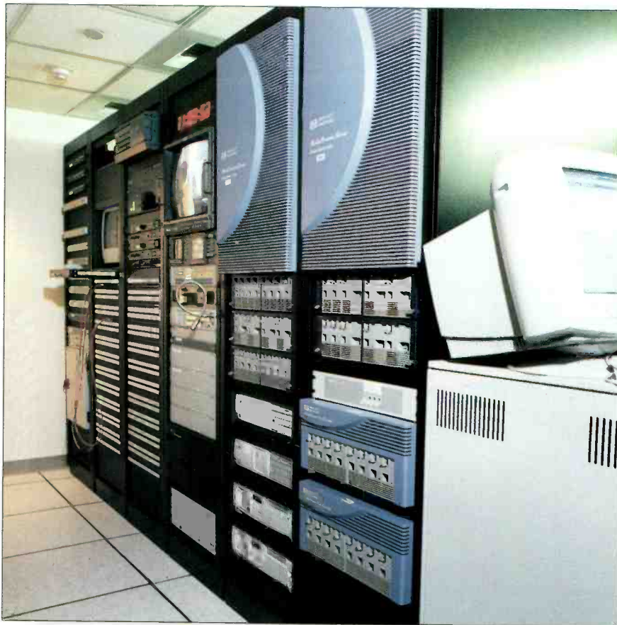
Lifetime's cart machines were replaced with video servers and disk arrays including these HP MediaStream servers.
