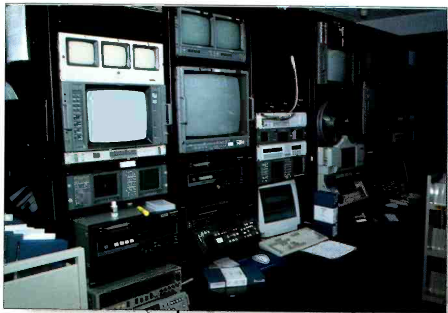
Ingest stations at Lifetime are used to turn tape-based spots and programs into disk-based files.
