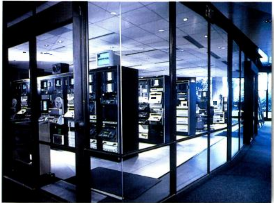
The Post Logic machine room.
