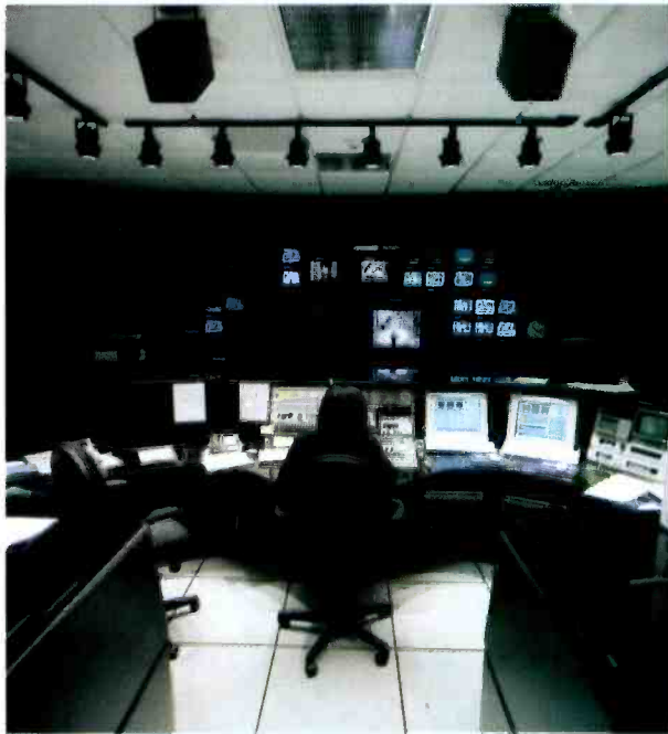
The master control room with a Philips Media Pool that is used for spot payout.
