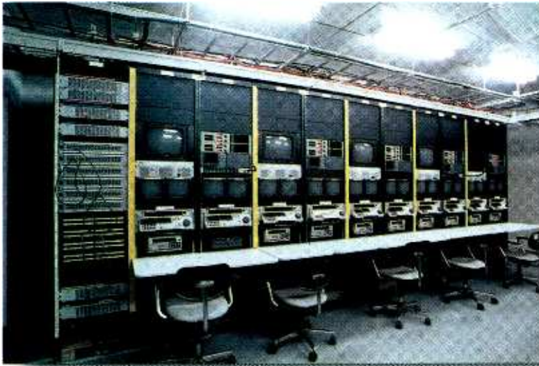
VTR room for archiving/library (IBC).
