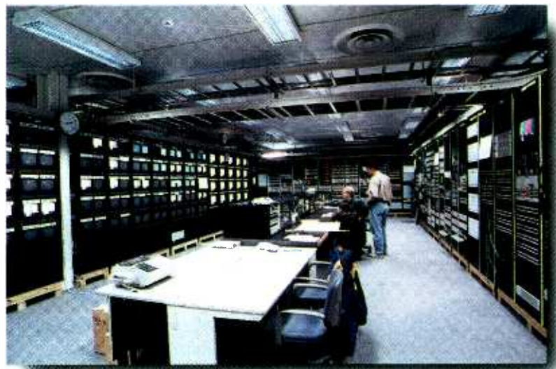
Distribution center inside of IBC.
