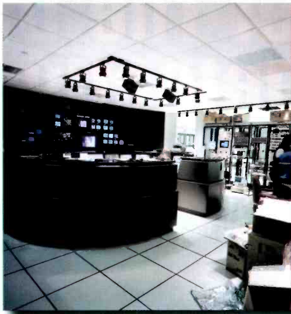
The master control room with an Itelco transmitter remote control shown in the background.
