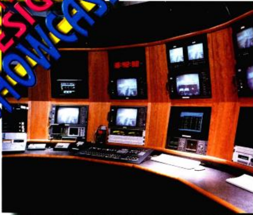
On-air switching is done with the BTS Philips Saturn digital switcher. This switcher provides a path to automated, multichannel operations.
