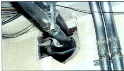
The packing blanket (labeled "trash") stuffed into gap around conduit will do little to attenuate noise passing through this oversized penetration.
