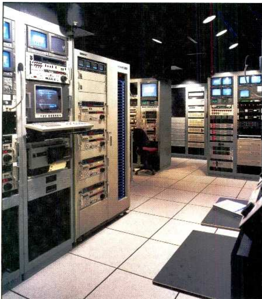
Modern automation equipment, complete with a library system, allows the network to operate by itself if desired. Shown here is the equipment area.
