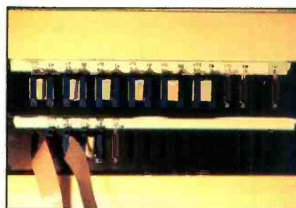
A digital patchbay made by using ribbon cable and press-on connectors. (Courtesy of Alan Wechsler.)
