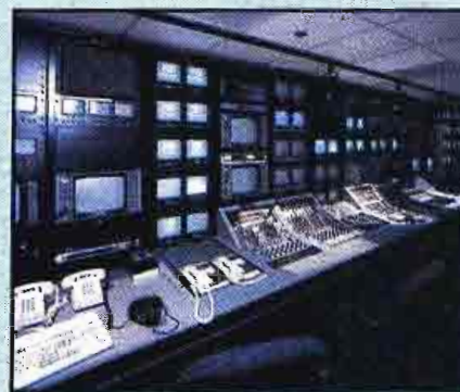
A portion of the subcontrol room showing the transmission and camera-control equipment. The video projectors and videowall also are controlled from this room.
