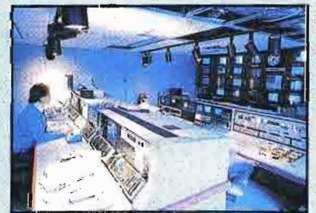
The WJLA-TV master-control room.
