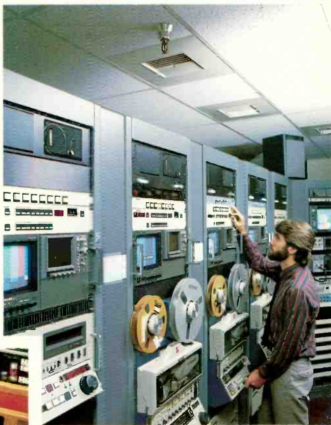
VTRs can be controlled with source selection panels and machine assignment panels.
