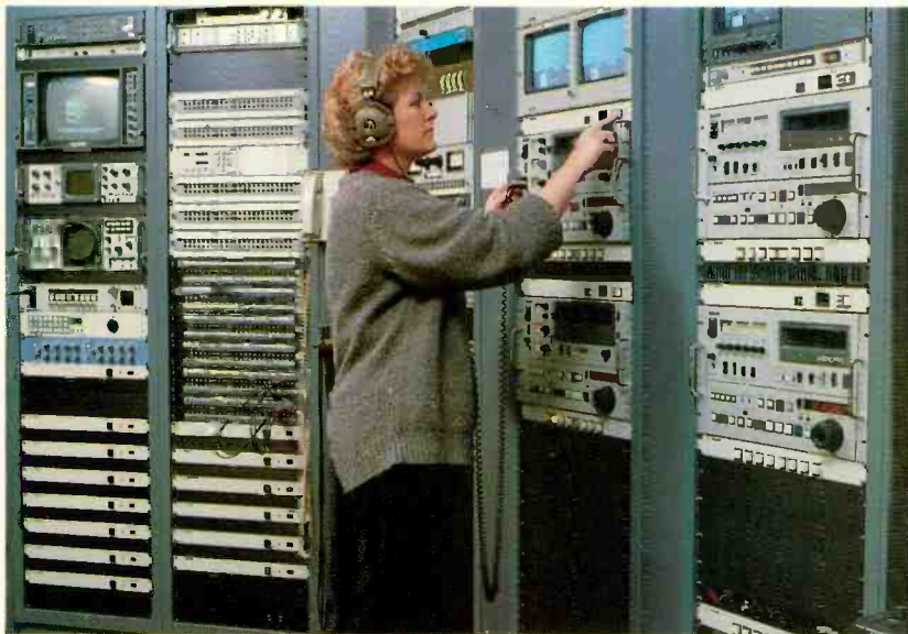
Machine control interfaces may be grouped together, or located at the individual machines.
