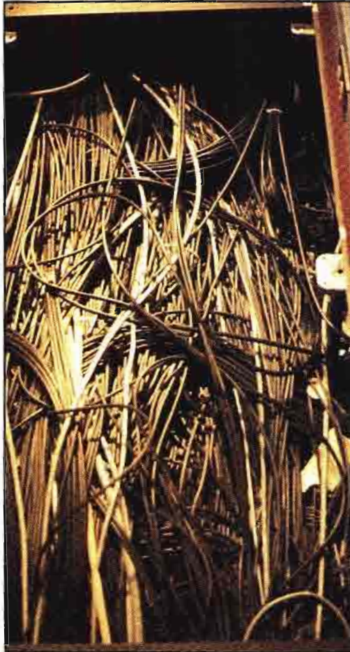
When determining raised-floor height, allow for extra-thick cable bundles around racks.
