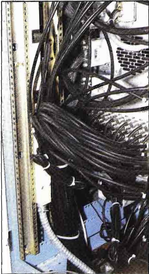
Delay lines are mounted on the rails of this production switcher rack.
