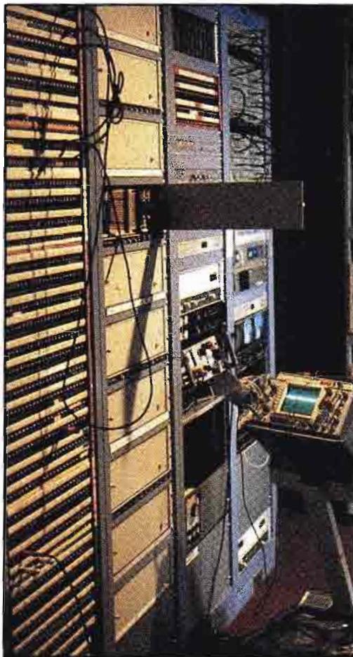
Placement of these audio racks allows easy access for maintenance.
