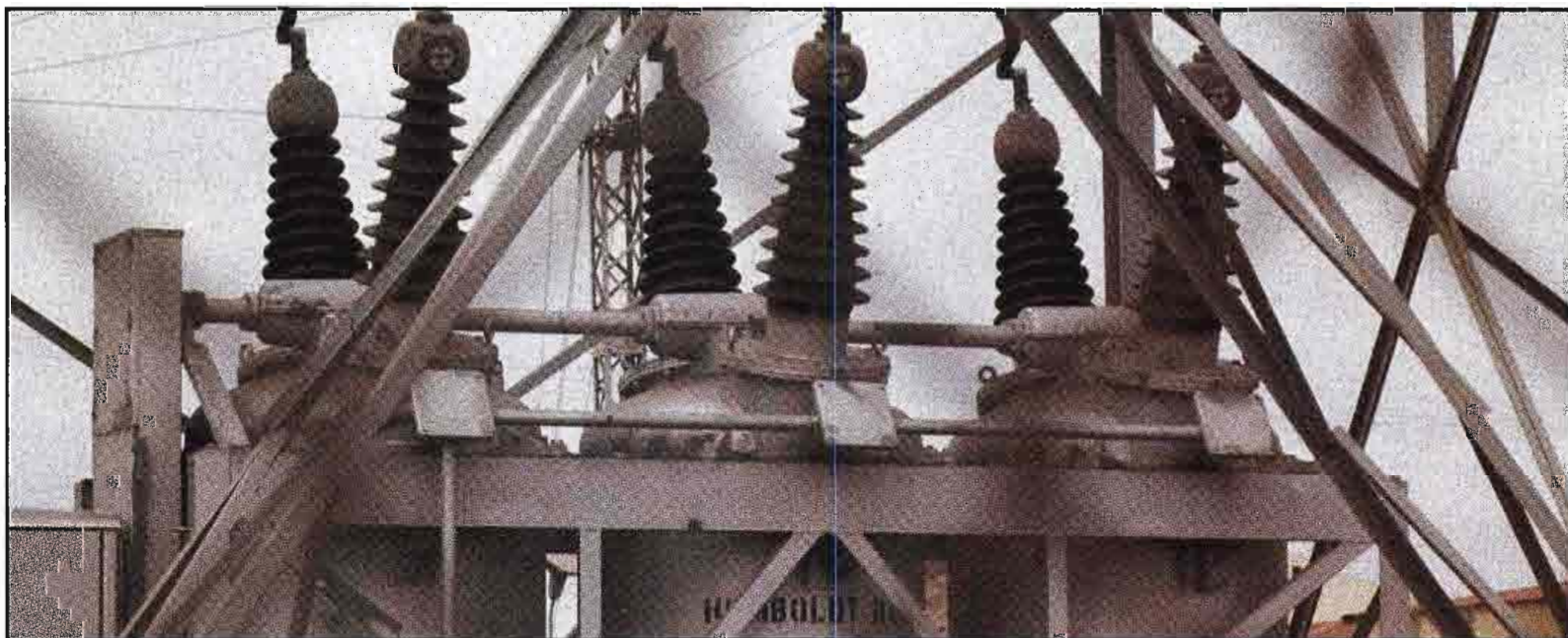
Disturbances on the ac power line into a broadcast facility can latch up or damage complex, sensitive equipment.
