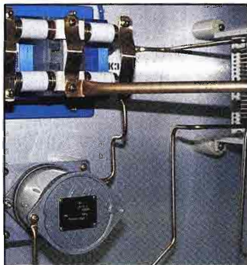
Inspect AM system antenna tuning units for loose connections or contaminants that could cause arcing.
