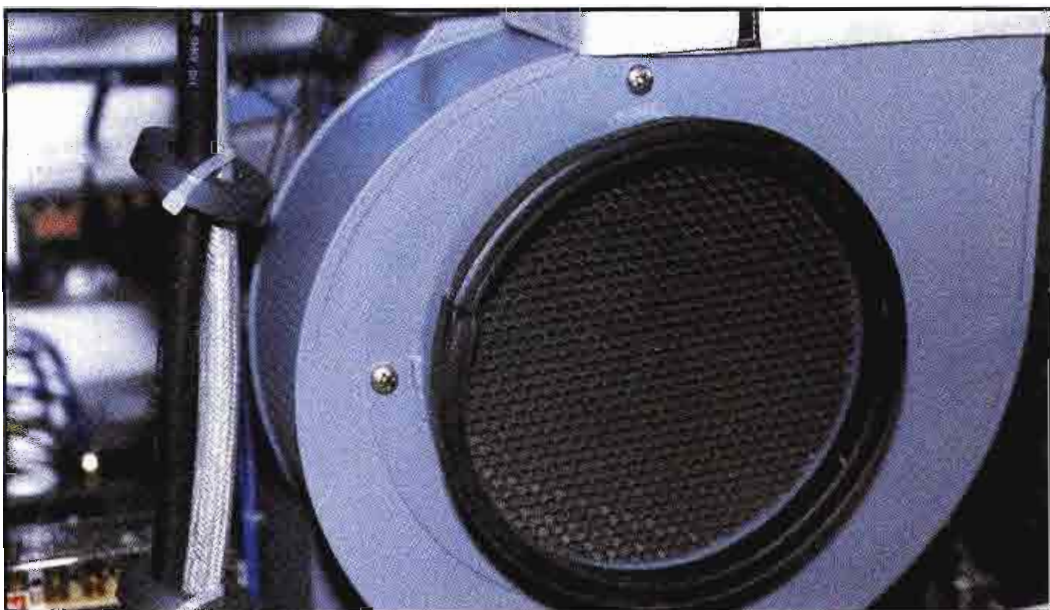
When troubleshooting a transmitter control ladder, don't forget to inspect the operation of the PA compartment air pressure switch and the associated blower assembly (shown here).
