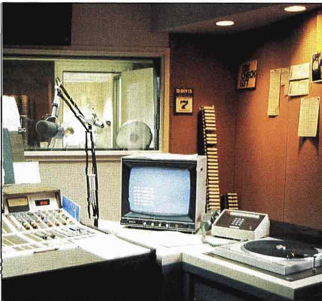
Control room lighting must illuminate the work surfaces (console) as well as other controls. If a CRT is located within the work area, it must not reflect glare from the lighting source.
