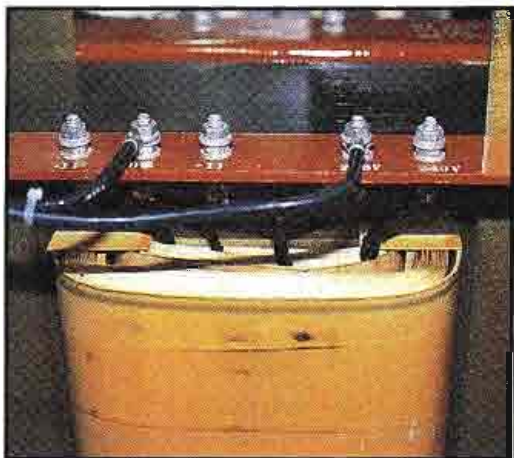
Don't overlook the obvious. Check the tightness of high-voltage and/or high-current cable connections.
