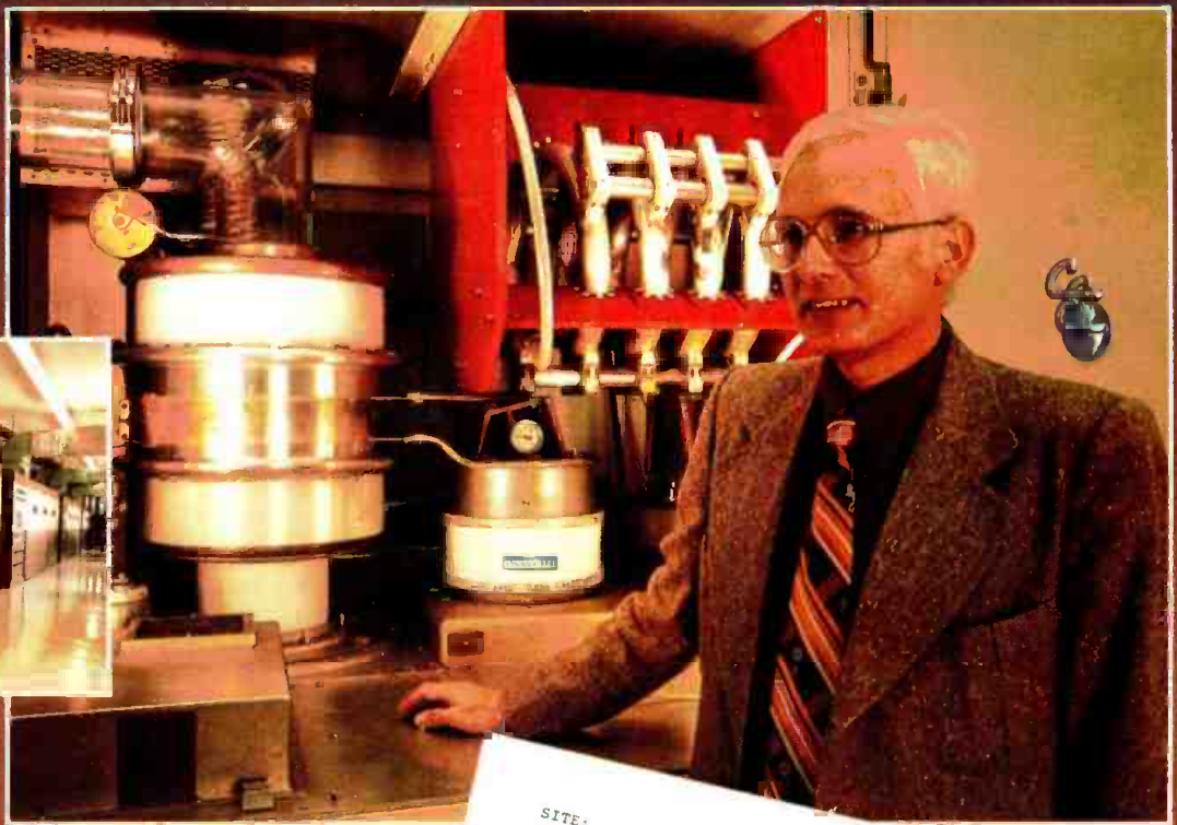
Hugh Falls, VP Engineering, Radio Free Europe, Munich, stands beside CE 100 kW HF transmitter using EIMAC 4CV100,000C tube.
