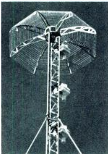
LEA LIGHTNING BARRIER. Typical Hemispherical Dissipation Array in use at a broadcast site.
