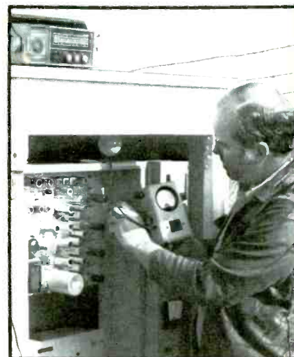
The author makes final adjustments at the Shadow Mountain antenna/transmitter site.
