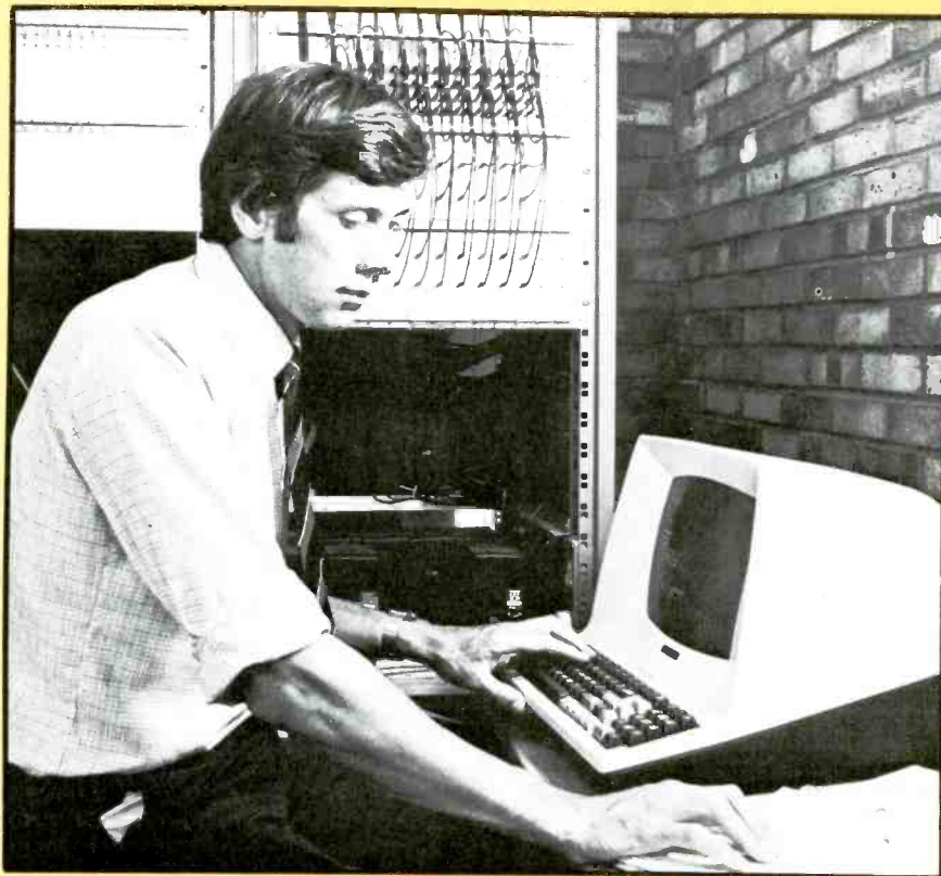
At the Milton Keynes flexibility point, in a small brick structure, a British Telecom research engineer uses the visual display unit to access the microprocessor unit (on left panel at rear) controlling the wideband switch (right panel), which channels the selected programs into customers' homes.
