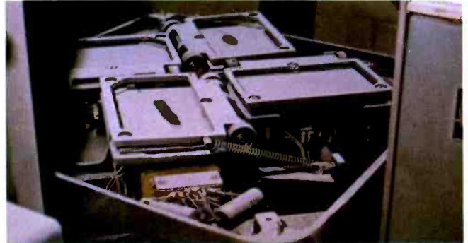
When the cover was removed from FC#2, a thick layer of powder was found on all surfaces. This chemical powder destroyed all plated optical surfaces. This photo demonstrates the appearance of the inside of all equipment in the telecine room.
