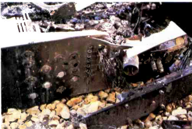
Rear connector panel of tape deck. The rocks under the panel are the remains of the concrete floor.
