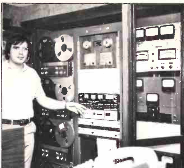
Tape decks, antenna monitor, EBS monitor, extended meter panel and other audio processing equipment in the main studio are behind two double-fold doors. Access also is available from behind and outside of the studio.
