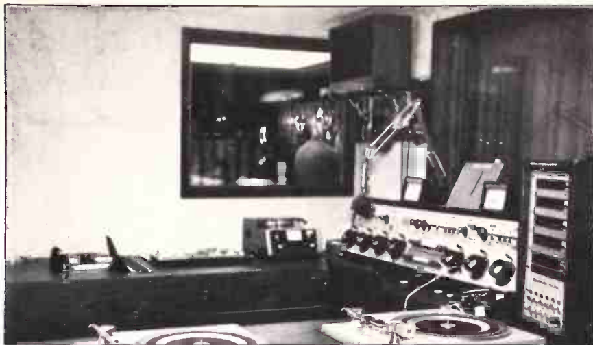
Studio B's layout is similar to the control room (visible through the window). Three hinged covers provide access to the patch panel next to the recorder while keeping dirt and debris out when not in use.
