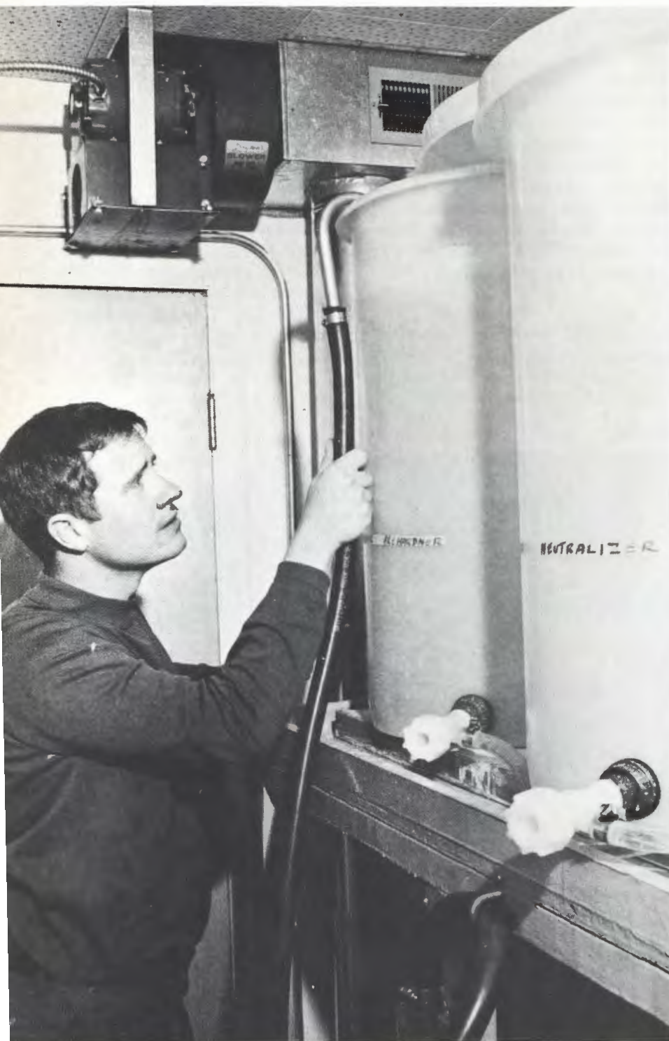
Fig. 2 KID-TV's Paul Jenkins shows method used to fill the storage tanks. The trays are made of fiberglass wood. Each tray must be capable of supporting at least 800 lbs. The ceiling mounted blower is for chemical mixer and storage room ventilation.
