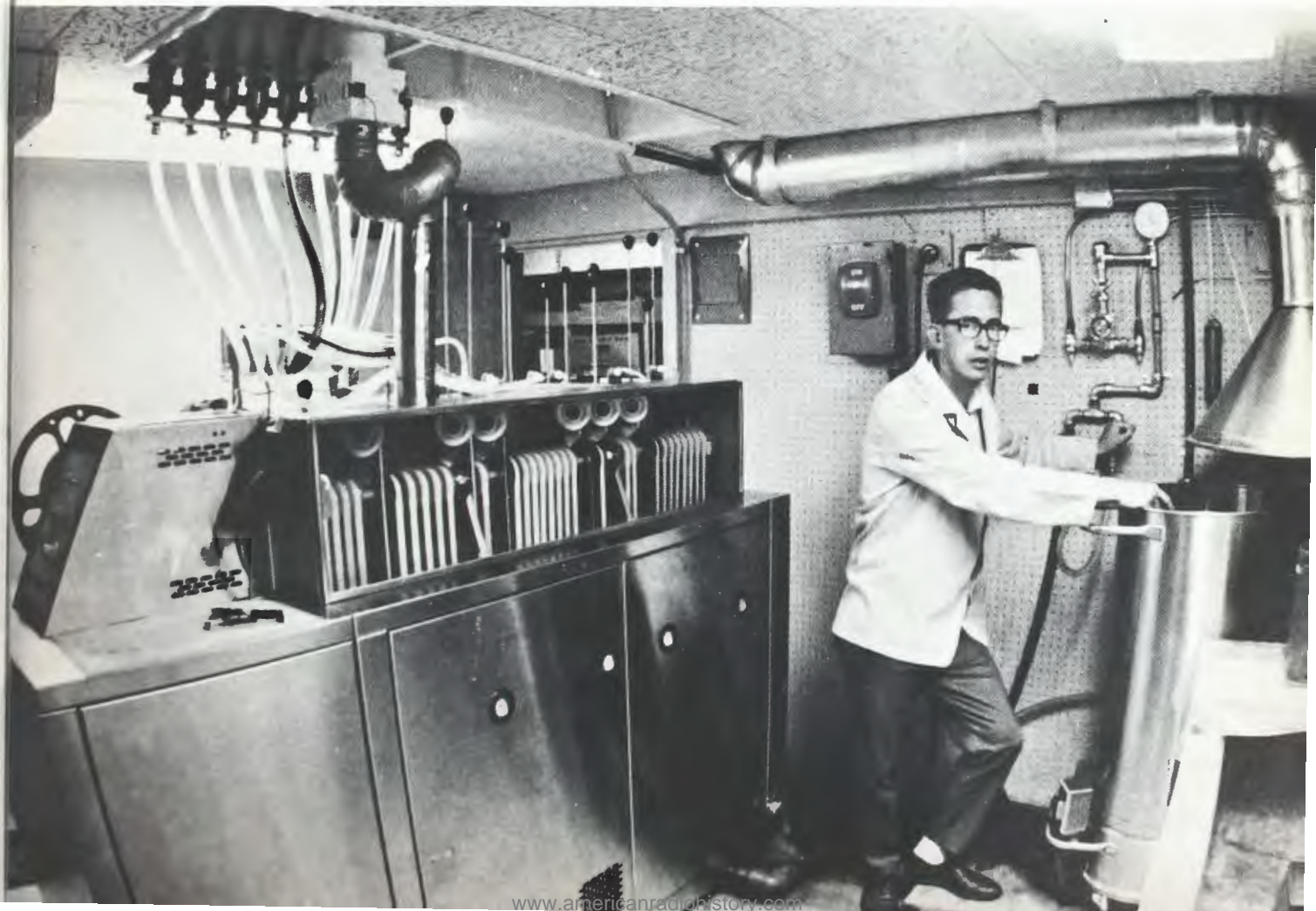
Fig. 1 KID-TV color processor installation with operator preparing to mix chemicals. Note cutout in ceiling to accommodate film transport rods. Replenishing lines and exhaust duct also run through the cutout.
