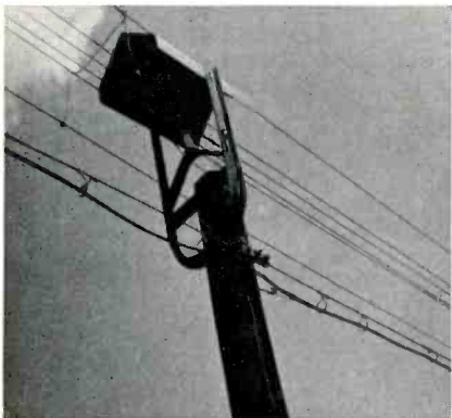
Fig. 3. View of frame atop one pole shows metal shield to keep ice off insulator.
