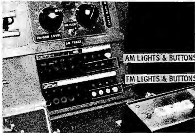
Fig. 1. Control panel placed in console.
