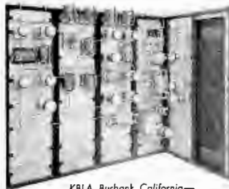
KBLA, Burbank, California— Six Tower, 10 KW, DA-2 Phasor.
