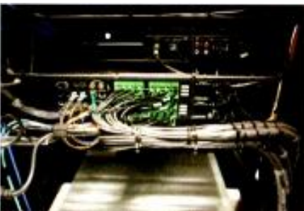
Shown here is an example of multiple copper-based signals combined onto a unified fiber-optic routing and transmission platform.
