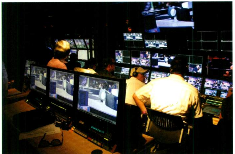
Inside the AMP 3-D truck, Sony MPE200 stereo processors are used to control the stereo images.
