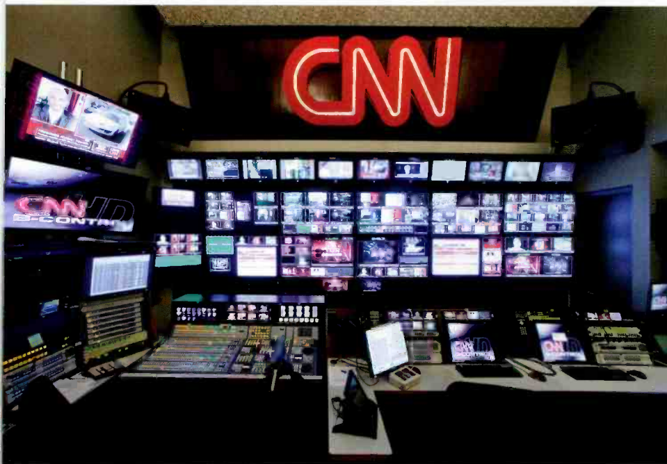
All new segments for HLN and other programs shot in the new studio will come out of Control B, complete with a Sony MVS-8000G HD production switcher and a multiscreen monitor wall running Evertz MVP multiviewer software.
