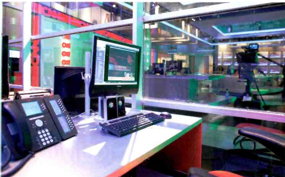
An internal IPTV network allows producers, journalists, editors and engineers to view a variety of live TV channels and incoming feeds from any computer in the building.
