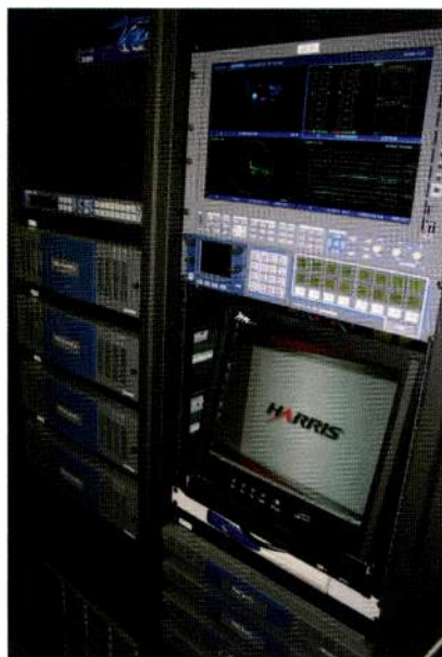
The facility includes three Harris NEXIO AMP SD/HD servers configured as a SAN.
