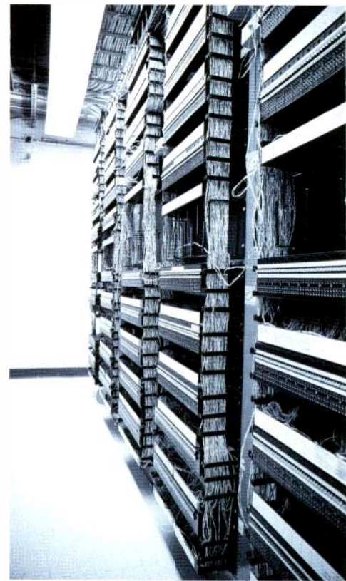
Fiber connectivity both between and inside broadcast facilities is now commonplace.
