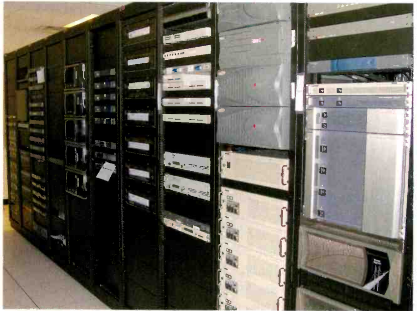
The 841sq-ft technical core contains 40 36-in deep racks, with expansion space for an additional eight racks.
