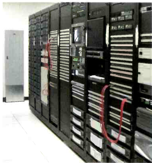
About 90 percent of the newsroom and all of the technical areas sit on an 18in raised computer floor.
