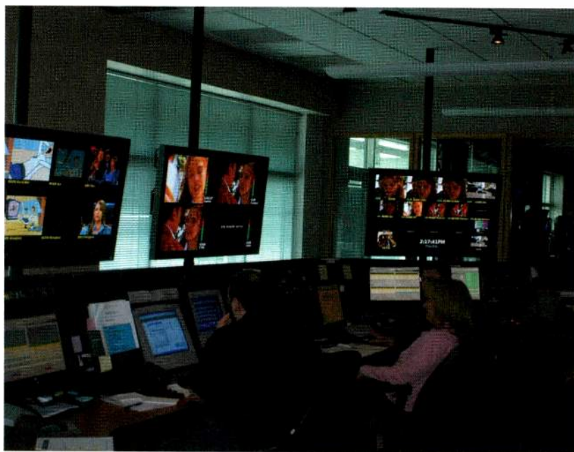
Using multiview monitors in a master control room enables multiple video signals for each station to be displayed on large-screen monitors.
