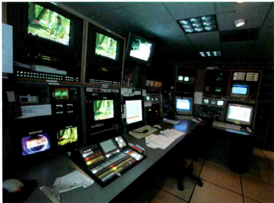
At the heart of NECN's network MC, a Utah Scientific MCP-2020 MC switcher, a Harris Leitch Panacea router and a SeaChange MediaCluster server system — all under Sundance NXT automation control — manage main program and dual-zone commercial content.
