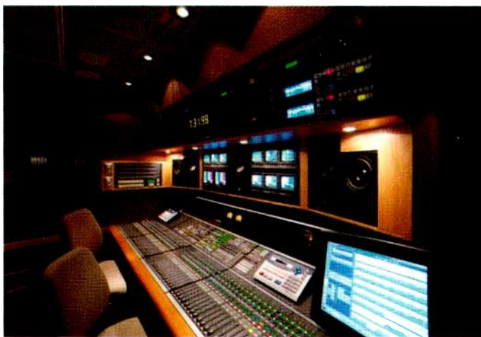
Game Creek Video installed a Sigma console in its Freedom HD truck. The console features Calrec's Bluefin high-density signal processing system, which provides more than double the processing power in less physical space.
