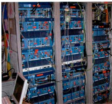
T-Systems ATM Broadcast Installations while the Olympic Games 2004 in Athens
