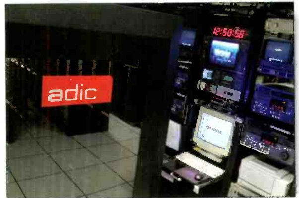
The station's automation system includes the LAN, ADIC archive and a SeaChange storage array.
