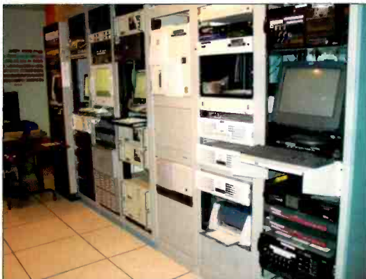
The central apparatus room features legacy Quantel Picturebox still stores and a Paintbox Express (in the foreground) alongside the new sQ server, editing hardware and new-generation Paintbox.
