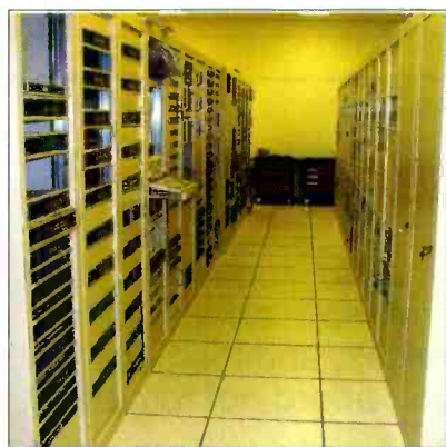
Many of today's rack spaces more closely resemble dense LAN installations than traditional analog distribution centers.
