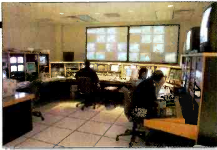
The technical operations center at Atlanta's WGCL-TV combines master control operations with news support to establish smooth workflow between the two operations.
