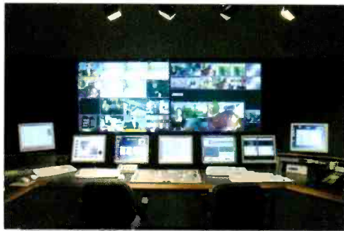
The master control room manages automation and command and control system monitoring for four DTV channels, four streaming channels and eight channels of satellite ingest.
